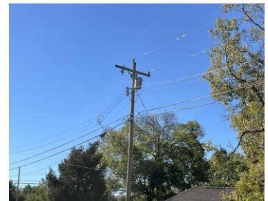
Currently pole mounted step-down transformers supply power to the street properties.
