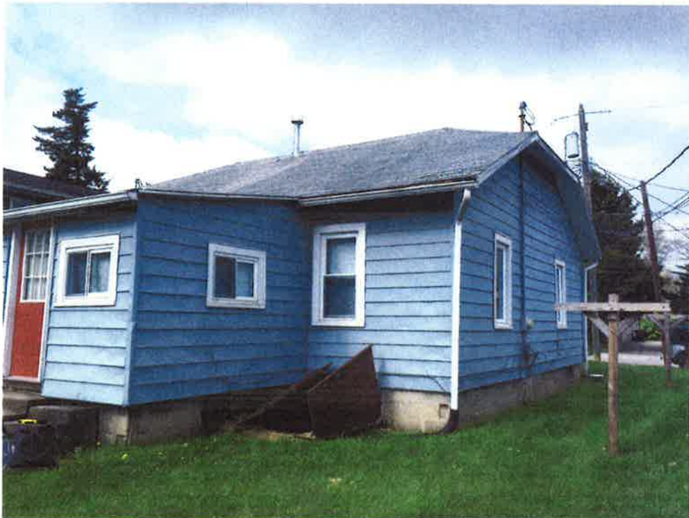
Rear of existing residence showing porch enclosure to be removed & exterior basement access to be enclosed
