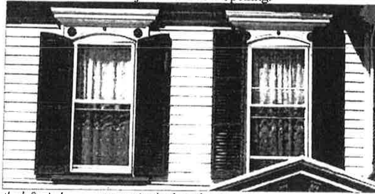
The shutters on the left window are appropriately shaped and sized for the related window even if they are not operable. The replacement shutters on the right are not appropriate due to the length and shape that do not correlate to the related window.
