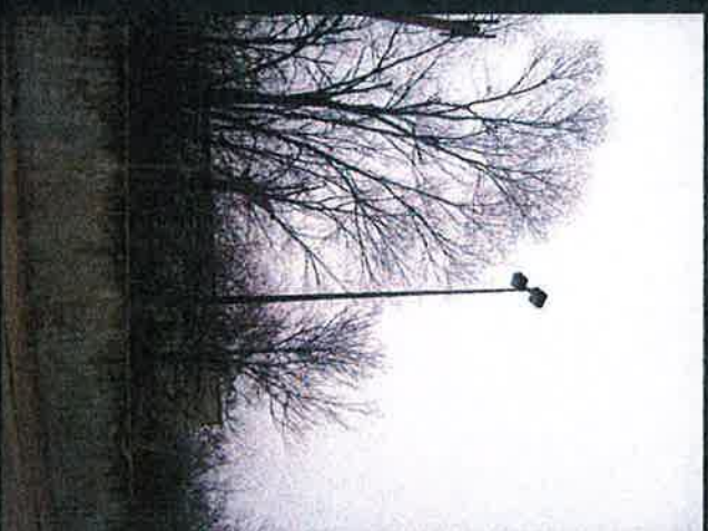
Existing Pole Lights at Property Perimeter
