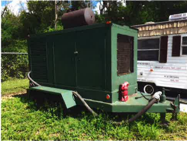
#11 1980 Cummins Portable Back-up Generator (No longer operational)
