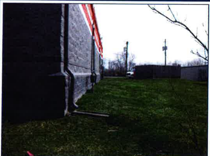
7 - Gas Service Behind Auto Zone
