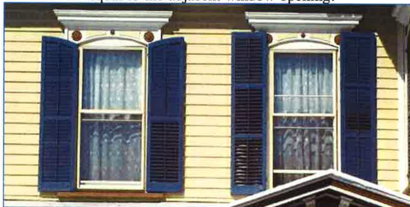
The shutters on the left window are appropriately shaped and sized for the related window even if they are not operable. The replacement shutters on the right are not appropriate due to the length and shape that do not correlate to the related window.
