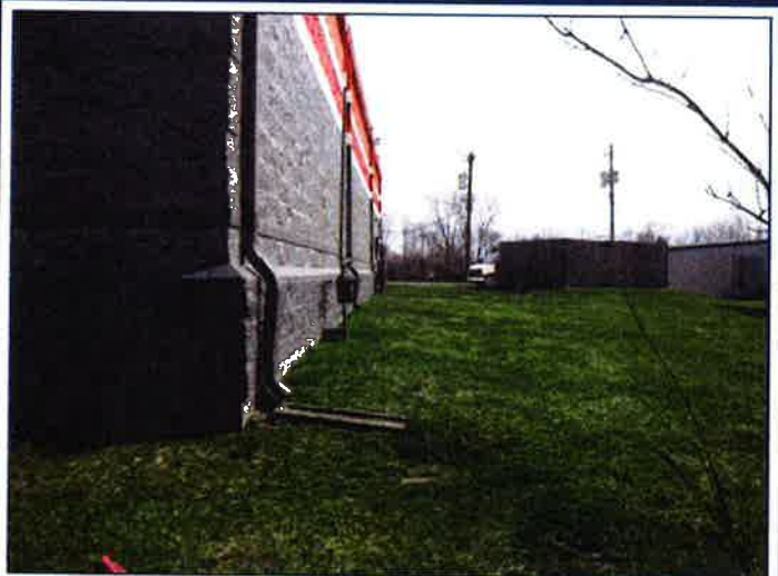
7 - Gas Service Behind Auto Zone
