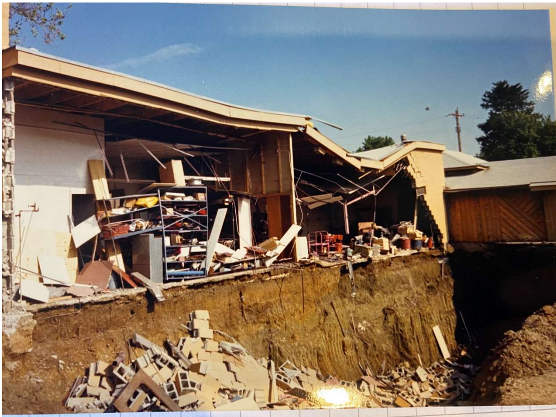
Partial collapse of east face of connector building during east lot excavation
