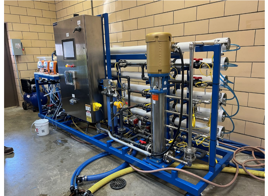
Membrane pilot unit
