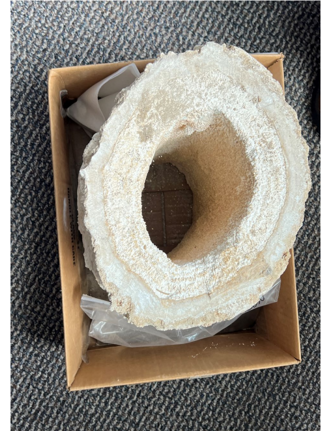
Scale buildup pulled from pipe with hard water
