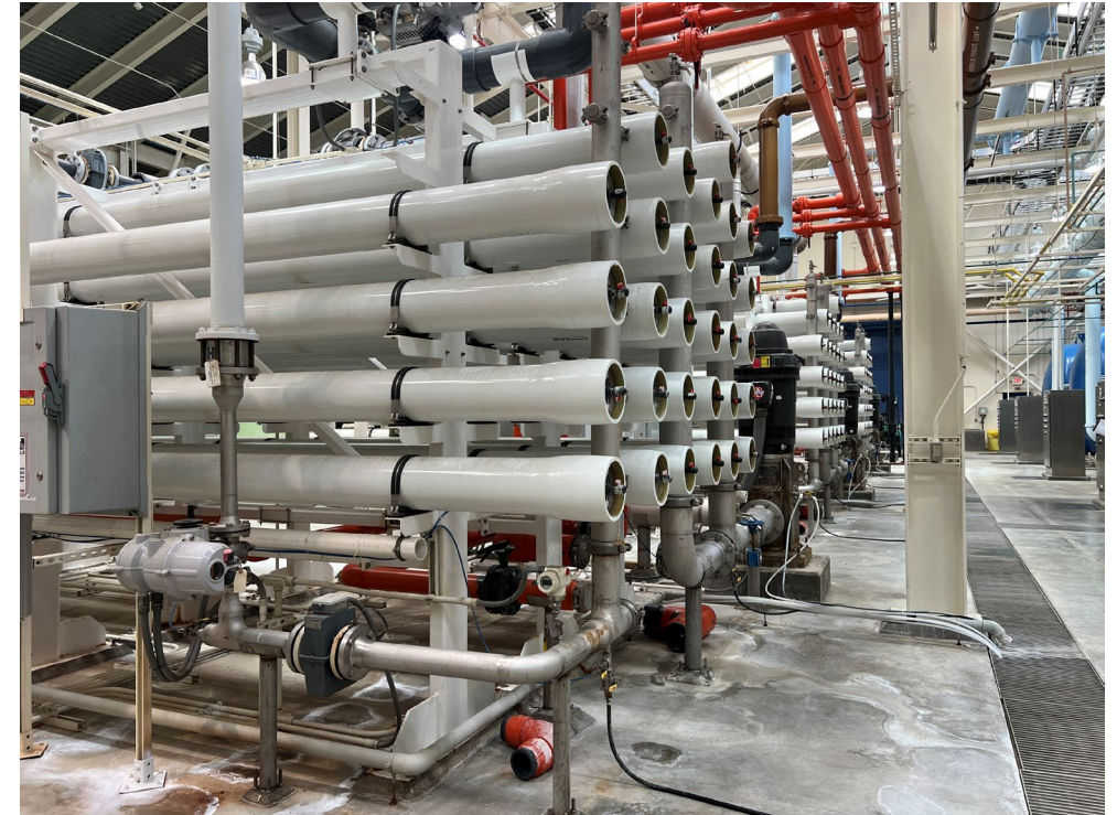
Membrane softening skid
