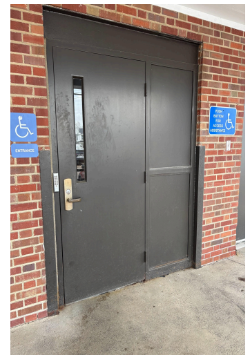
Accessible door in the back of the building. The door can only be opened by the staff from the inside.
