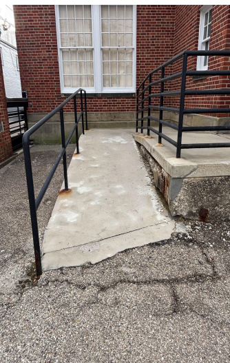
Uneven ramp that is covered in rocks and pebbles, making a difficult transition from the road. Additionally, the ramp is only wide enough for one person at a time, meaning people would have to walk in a line rather than next to each other.
