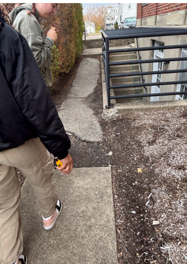
Uneven sidewalk on the side of the building closest to the curb cut. This makes it difficult or impossible for disabled people to access the accessible entrance from this side.
