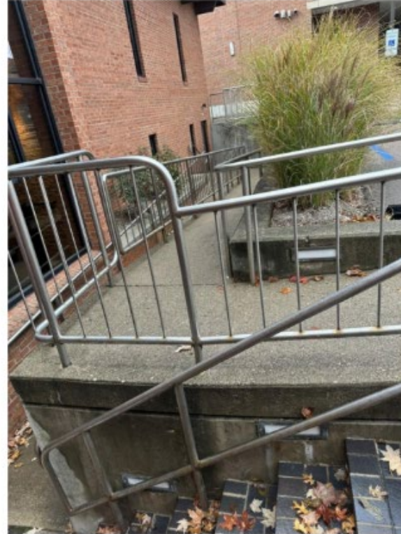
Image 1.4 *Image shows the ramp, at the entrance with the attached parking lot, with a ramp that has several narrow turns.
