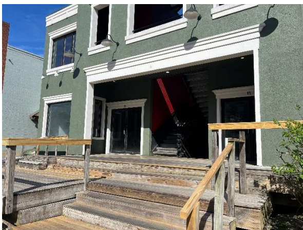
Wood Deck to be replaced
